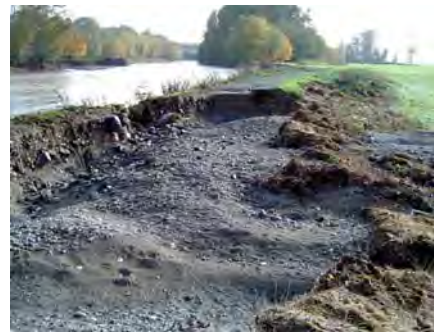
Figure 2.2 Flood damage. (WA)
