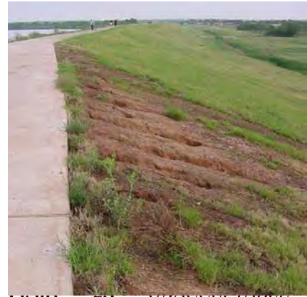
Figure 2.1 Erosion of levee slope. (TX)
