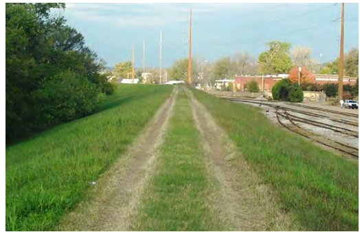
Figure 2.39 UNACCEPTABLE rutting in levee. (OK)
