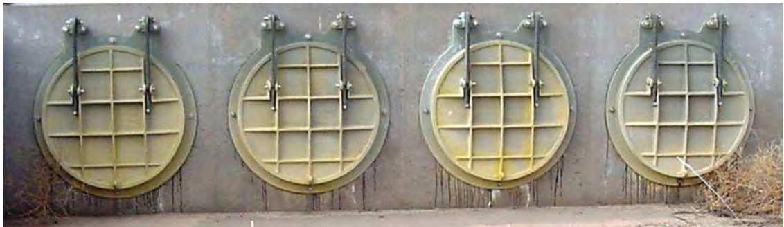
Figure 2.64 ACCEPTABLE flap gates in earthen levee. (KS)
