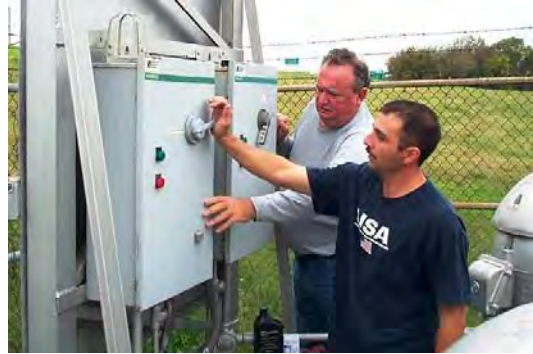
Figure 7.1. Inspection of pumping station controls. (OK)
