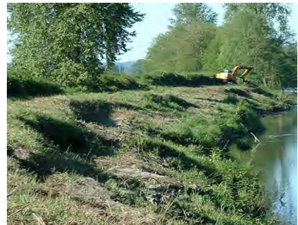
Figure 2.3 Slope failure on bank protection project. (WA)
