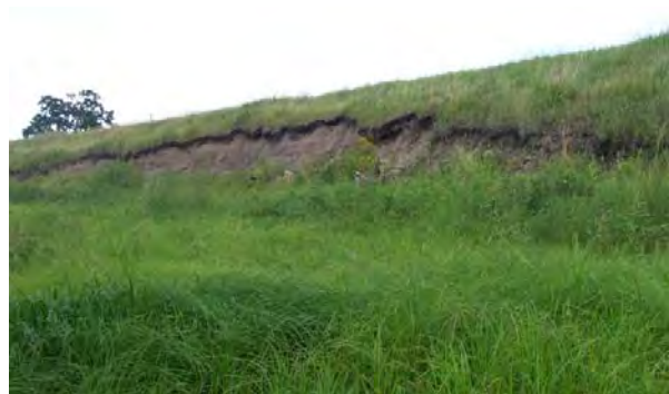
Figure 2.17 UNACCEPTABLE earthen embankment failure. (MN)
