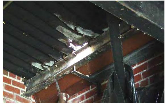
Figure 2.67 Hole in roof of pumping station. (IL)
