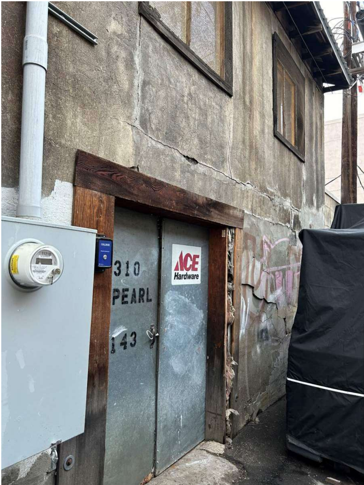
Looking northeast at the large cracks in the gray stucco siding, indicative of the bulging and deterioration of the east wall of the warehouse addition.
