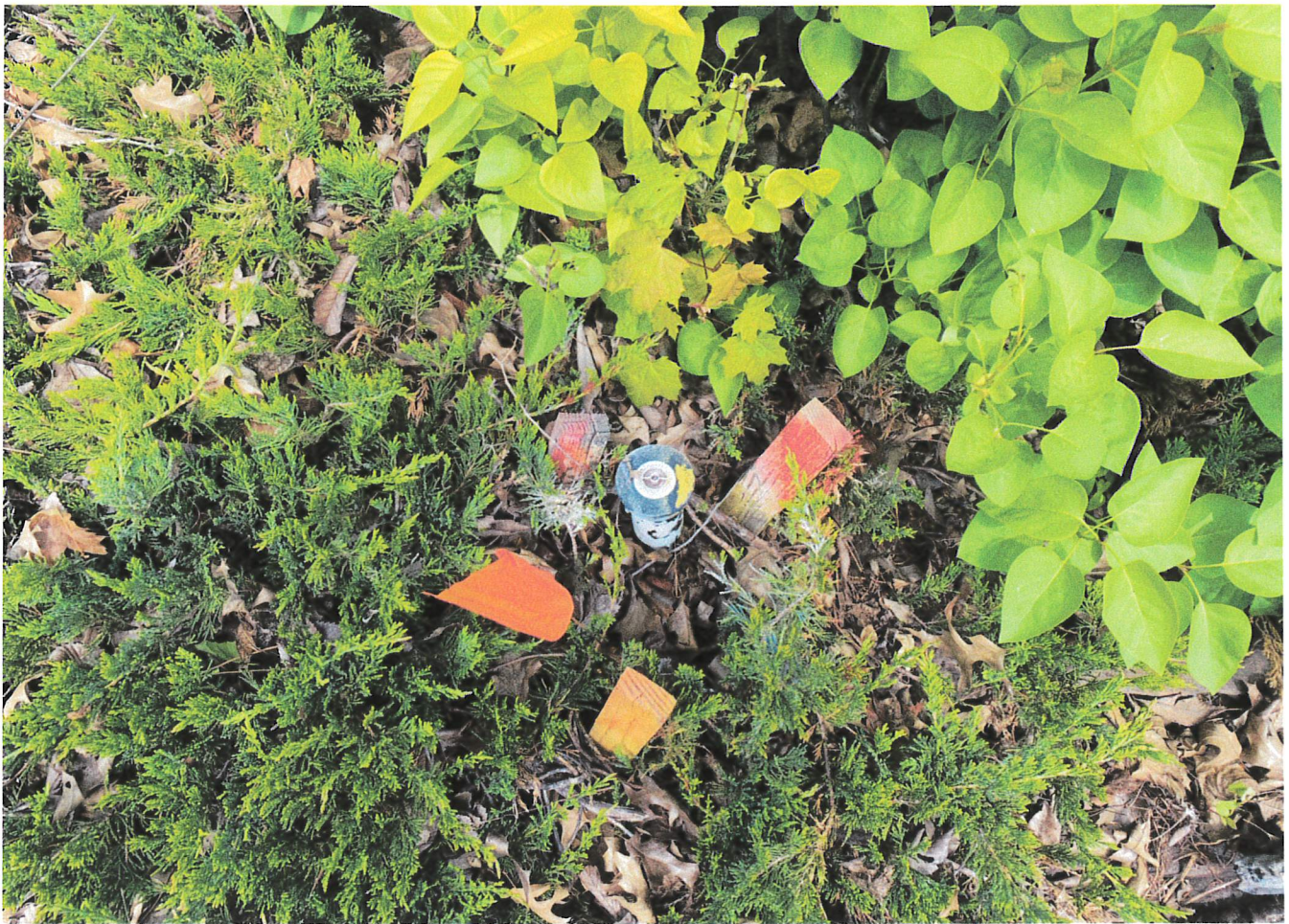
Close up sprinkler
