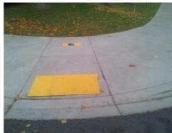
B Category Nearly Compliant
