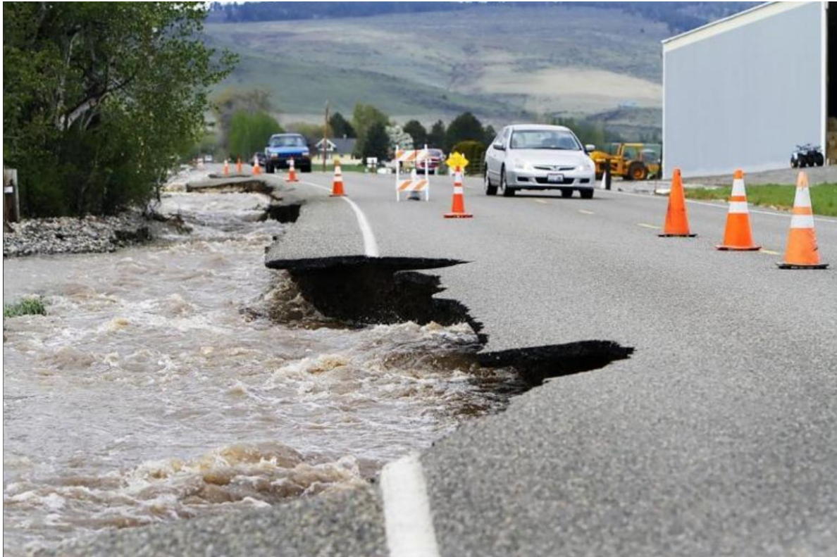
Figure 10: Rushing flood waters near Manastash Creek where a portion of Hanson Road being washed away in May 2011.
