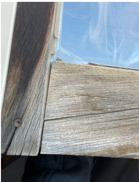
Exterior view of the existing window sashes and gaskets deteriorated condition.
