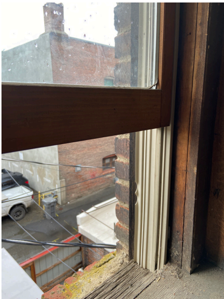
Close up view of the existing retrofit windows with wood sashes in vinyl tracks. The gasket around the glass can be seen separating from the corner.
